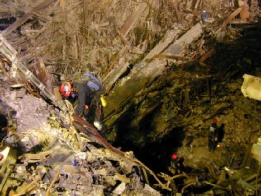
Figure 4-1 - GZ workers descend into the subbasements below WTC2. While there is extensive damage, there is little building debris at the bottom of the hole. There is no sign of molten metal. A worker in the distance walks along a massive core column. (photo filed 9/18/01) 86
